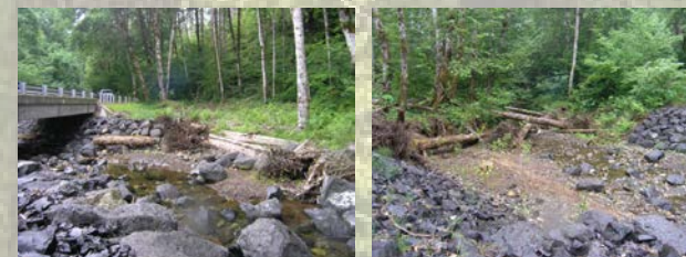
Examples of riparian restoration following a bridge replacement across a stream. A major objective of this project was the restoration of aquatic habitat. Old trees, complete with their root-balls, were maneuvered into position as coarse woody debris along the channel (photo left). Planting of riparian understory species was also undertaken for ecological enhancement and bank stabilization (photo right).
